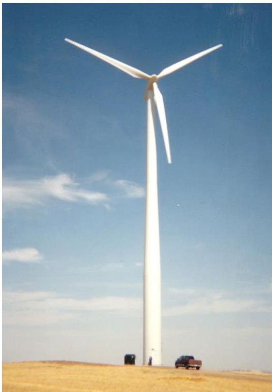
Horizontal Axis Wind Turbine (0.66 MW ac )
