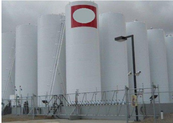
Welded Steel Tank
