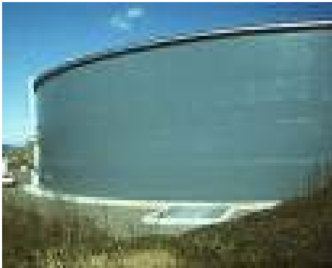
Welded Steel Tank
