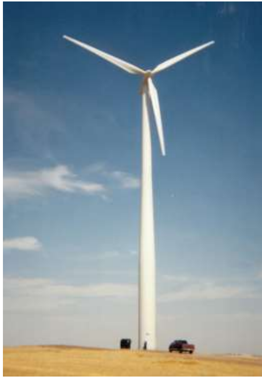
Horizontal Axis Wind Turbine (0.66 MW)
