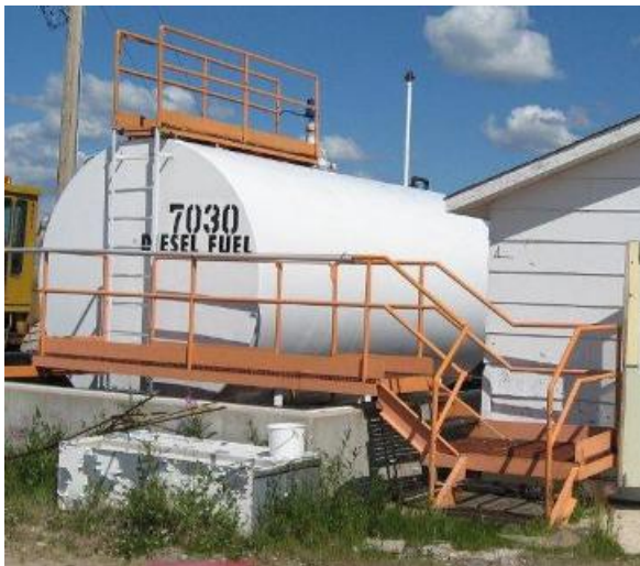
Steel Bulk Storage Tanks
