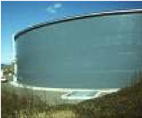
Welded Steel Tank
