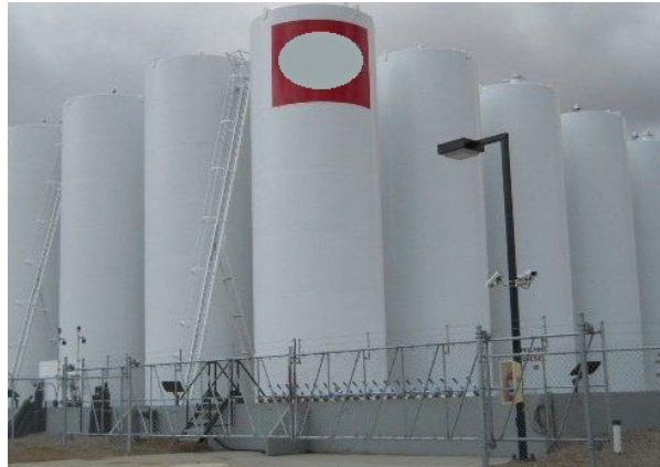
Welded Steel Tank
